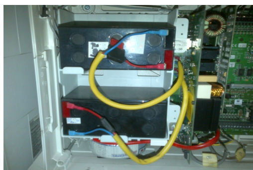
Gambar Battery Backup
